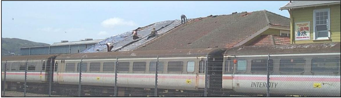
The heavy tiles were removed from the Railway Hall and replaced with black polythene
