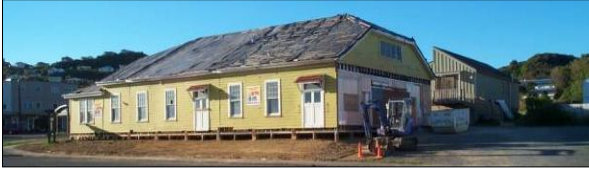
After the move from Moera to Maungaraki a new roof was the first priority
