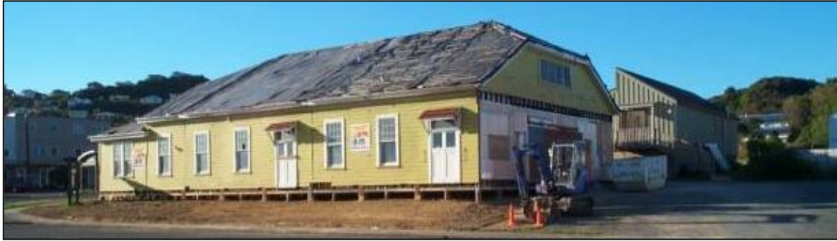
After the move from Moera to Maungaraki a new roof was the first priority
