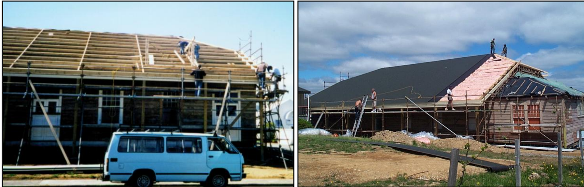
Building an 'ark'- being in a high wind zone meant that the roof had to be strengthened
