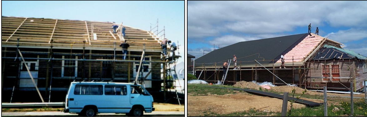
Building an 'ark'- being in a high wind zone meant that the roof had to be strengthened
