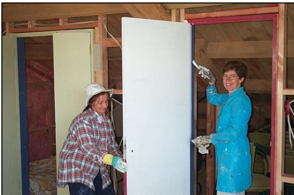
Fiona Coughlan and Priscilla from the Hope Centre painting the doors upstairs. On the right is one of the original doors after being stripped and polyurethaned.
