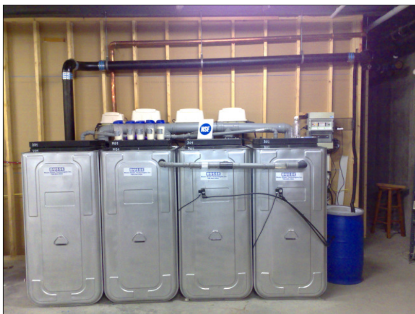
Installation of the system in the basement
