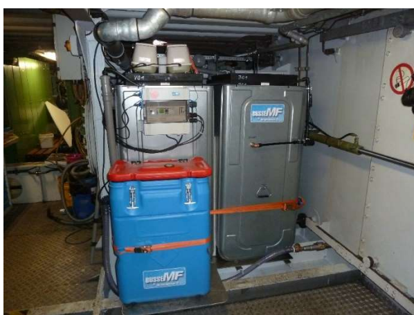
waste water treatment plant
