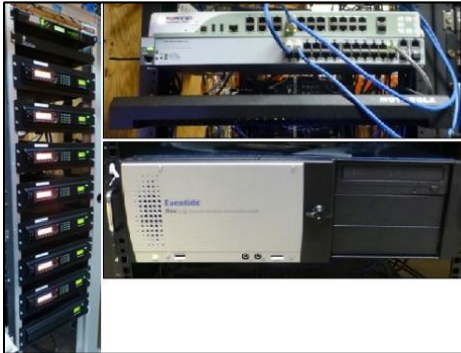
Central Dispatch Equipment.
