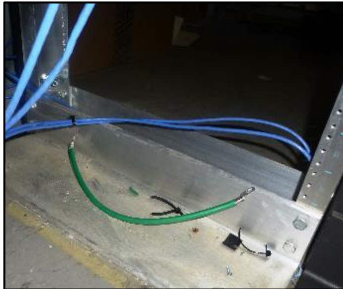
APX radio rack not bonded to ground
