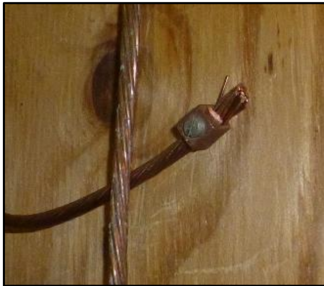
Example of ancillary equipment not bonded.
