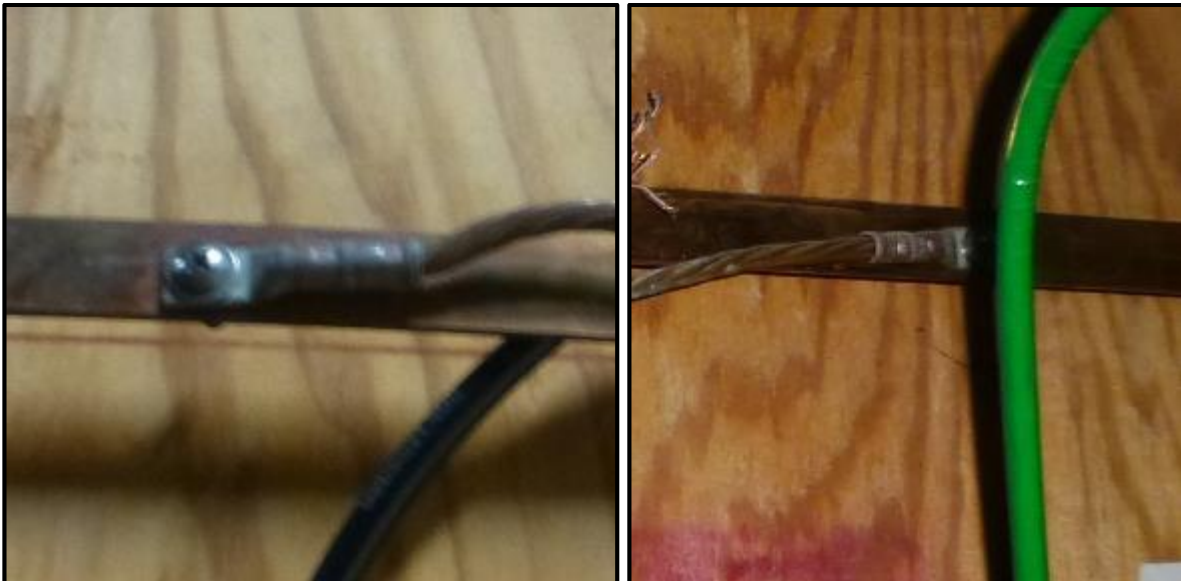
Examples of ancillary secured to the perimeter bus in the wrong direction.
