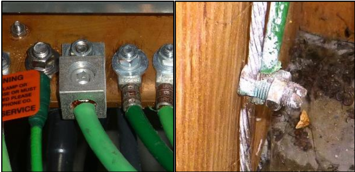
PBB earth grounding connection.
