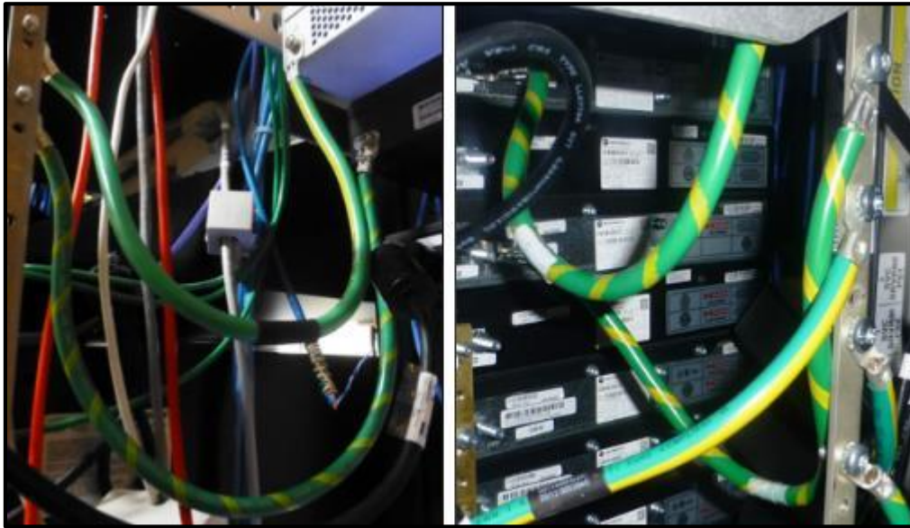
Bonding jumpers exceed minimum bending and routing requirements.
