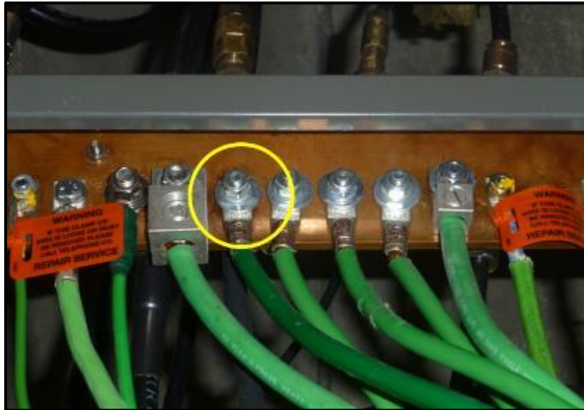
Connections to the equipment room PBB.
