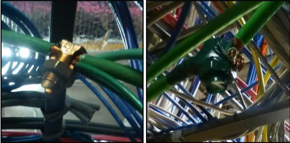
Multiple pieces of existing equipment secured to bus conductors with split bolts.
