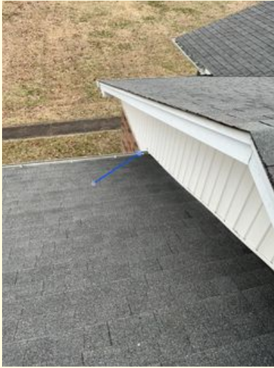
Missing kick out flashing
