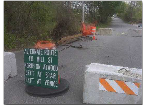
Figure 2: Mill Street closed due to flooding on March 31st, 2010
