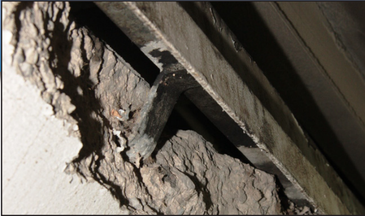
DAMAGE CAUSED BY BUSES
