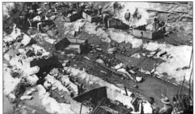
Extensive excavation was required before dam construction could begin. Hundreds of workers from outside the county came in during periods of construction
