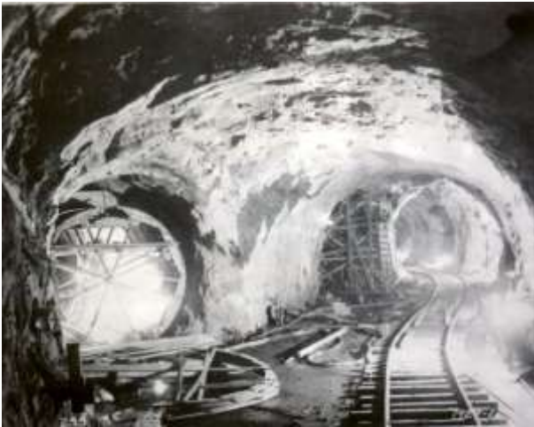
Calderwood Penstock Tunnel drilled during construction of the Calderwood Dam in 1929. (Greg McClain/Knoxville News Sentinel)
