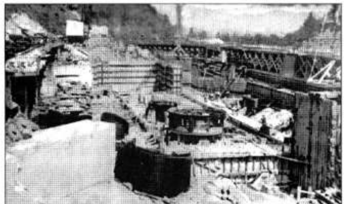
Large generators were set in place to produce energy to Alcoa's Tennessee Aluminum Facility
