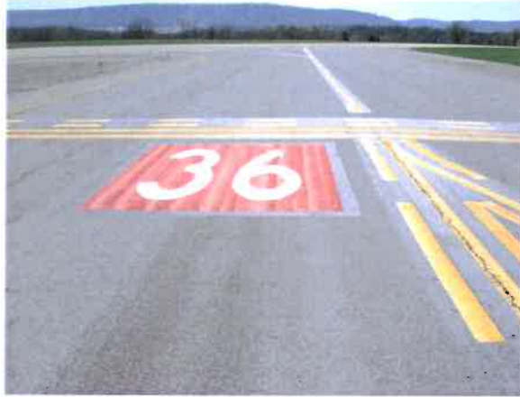
Surface painted hold sign on Txy A at Rwy 36 approach
