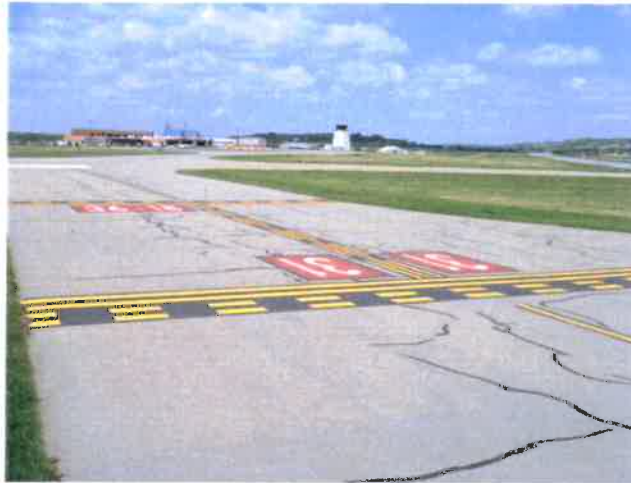
Double HOLD lines on Txy B between Rwy 31 and 36 Note: Make sure you are located at the proper hold line!
