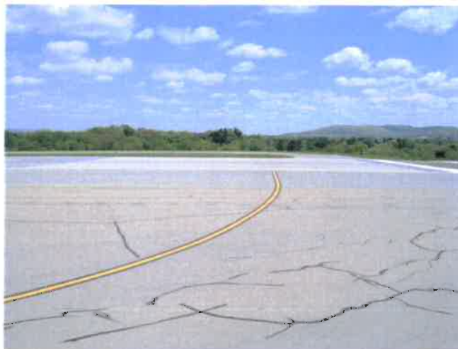
Taxiway lead-in line and Threshold bars located at Rwy 31 approach end
