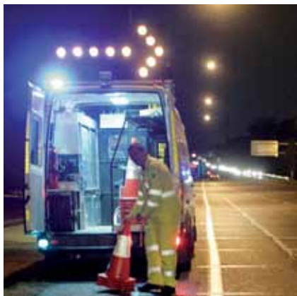
Road hazard ahead. Merge lanes.
