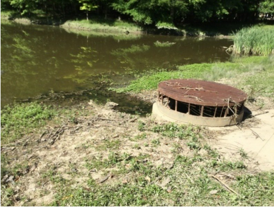
View of debris accumulation at the outlet structure.
