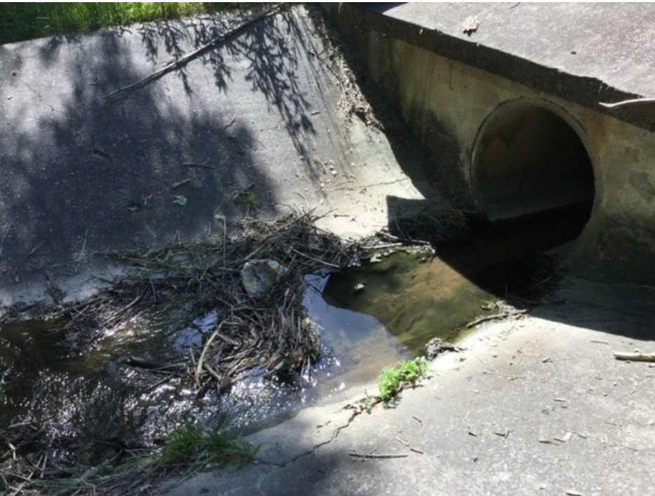
View of debris accumulation at outlet structure.
