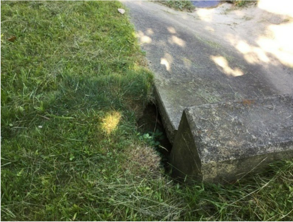
View of erosion occurring at the headwall (east).
