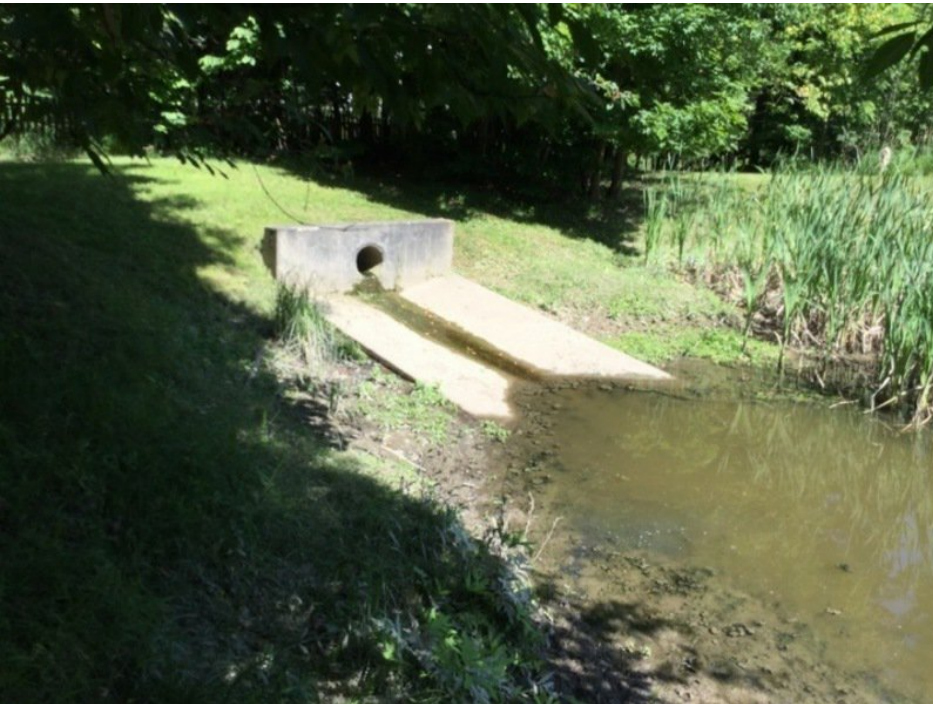
View of inflow structure in the northwest with sediment accumulation and invasive plants.
