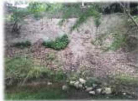
Steep eroded bank at 9836 Silverleaf
