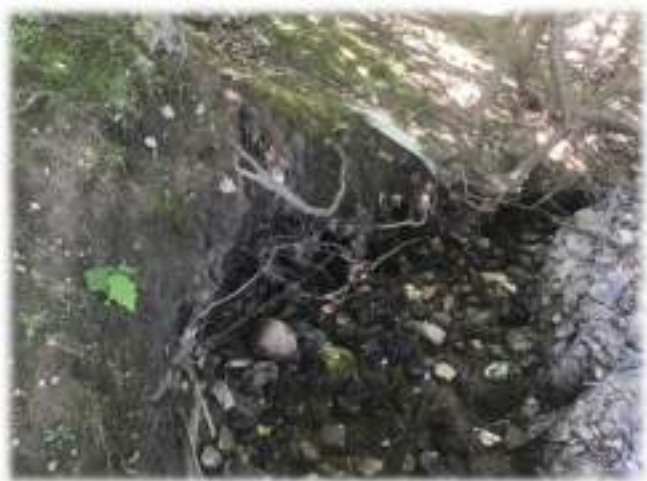
5031 Corkwood Drive- failed gabion baskets
