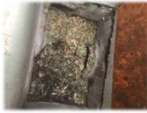
Catch basin debris- Sweetleaf Lane
