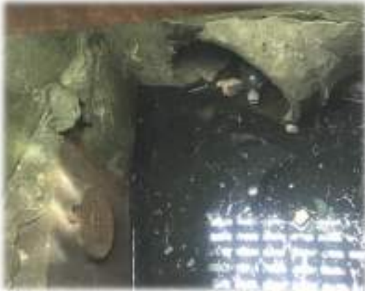
Circular orifice plate restriction- Corkwood Drive
