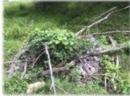
Failed gabion downstream of 5117 Pinckneya
