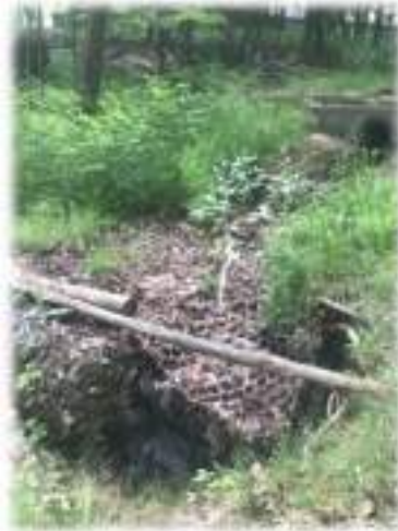
9780 Royal Valley Outfall
