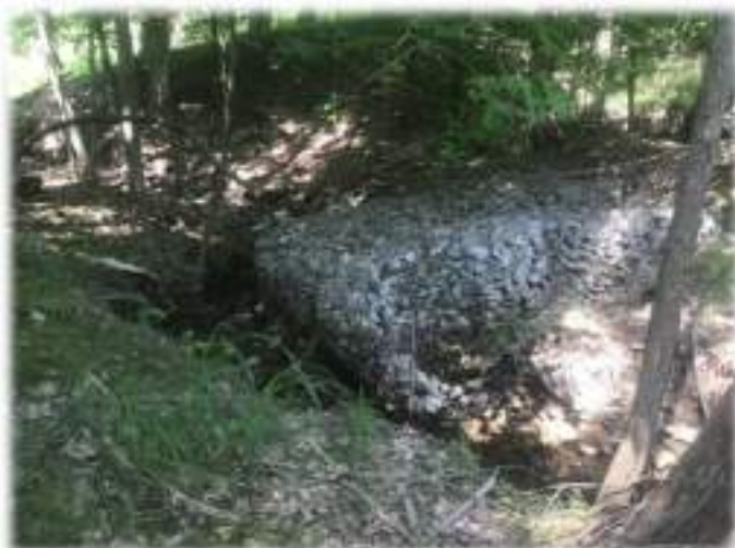
Failed perpendicular gabion feature, 5031 Corkwood Dr.
