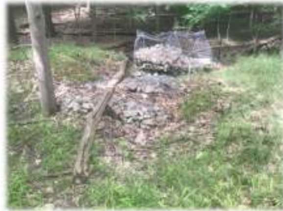
Failed Gabion structure within channel between Dublin Drive and Buttonbush Lane
