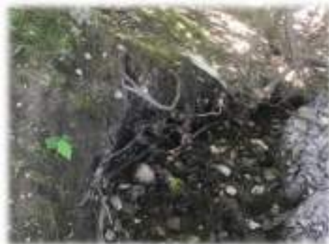
Failed gabion and bank erosion downstream of 5031 Corkwood Drive
