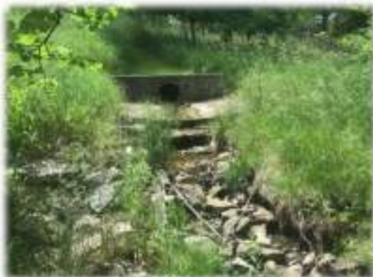
9769 Royal Valley Outfall
