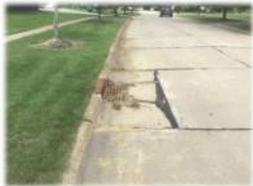
Roadway debris within gutter along Pickneya Drive
