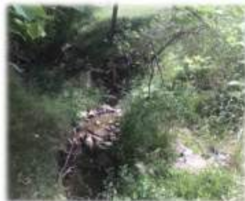
Downstream bank erosion at 9769 Royal Valley
