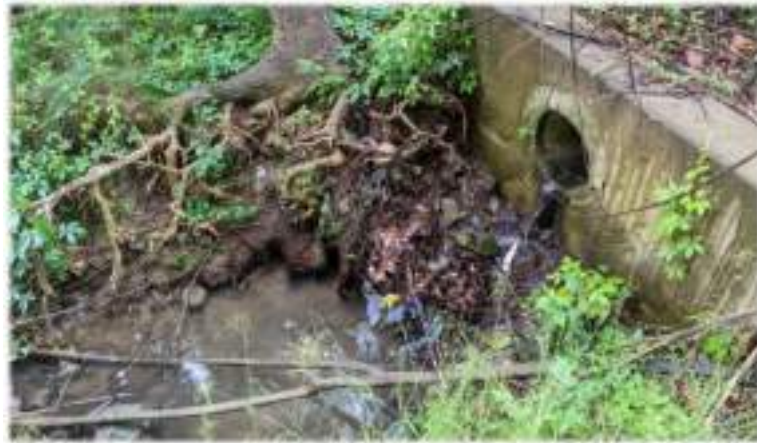
Outfall near 5117 Pinckneya Drive with 2-foot-deep scour pool
