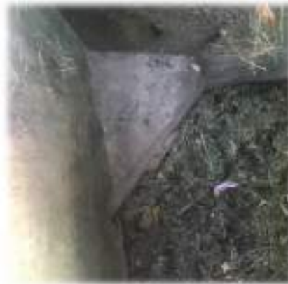
Catch basin debris with orifice restriction- Pickneya Drive
