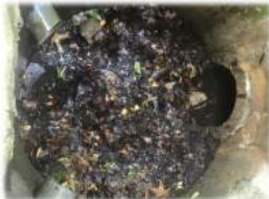
Catch basin debris- Ridge Line Drive
