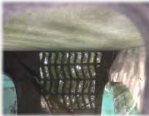
Inside of Inlet Basin 2 (IB2) from north showing an east and west pipe orientation.
