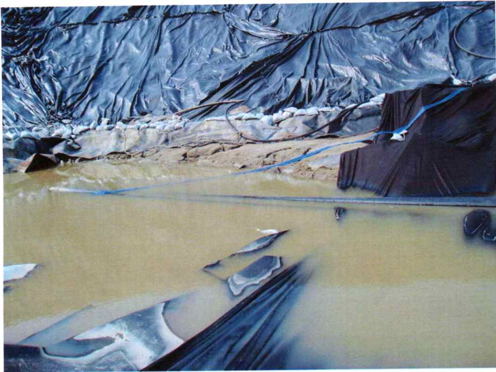
Contaminated storm water in Phase II Stage II sump and Phase IV berm notch.
