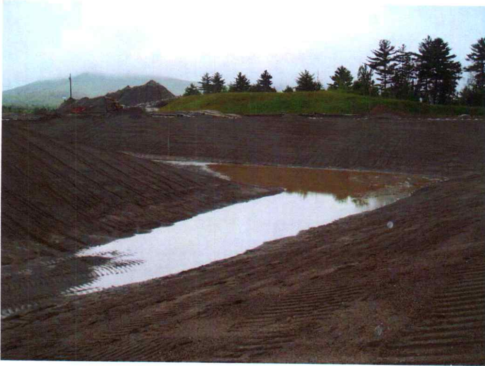
Contaminated storm water in Phase IV Stage I.
