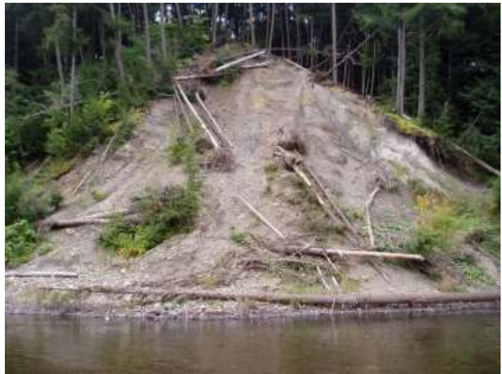
Riverbank erosion on the Ammonoosuc Photo by Field Geology Services, 2009
