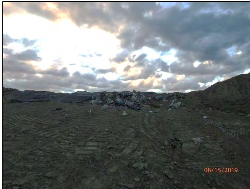
P8150008: Working face in the southern portion of Stage IV/Phase II, prior to the working face being uncovered, as viewed from the west and looking upslope in an easterly direction. Pile of soil cover mixed with debris present in the center of the photograph; pile of soil cover present on the right of the photograph.
