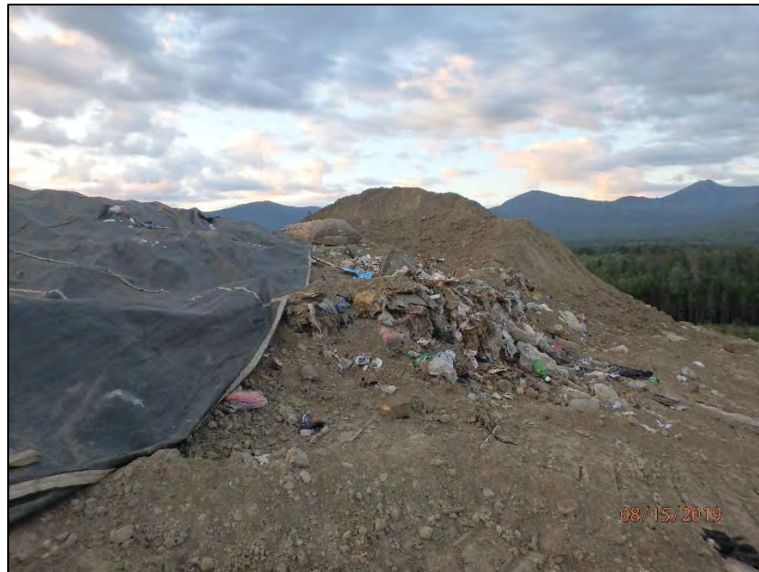
P8150006: Southern portion of Stage IV/Phase II, prior to the working face being uncovered. Looking south. Pile of soil cover mixed with debris present in the center of the photograph; pile of soil cover present in the background of the photograph.
