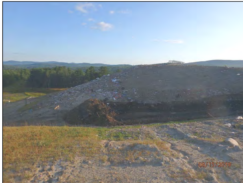
P8150025: Working face in the western portion of Stage V/Phase II, as viewed from the south. Prior to this photograph, NCES personnel removed a limited layer of cover material on the southern edge of the Stage V/Phase II working face to create room in which to deposit a load of sludge.
