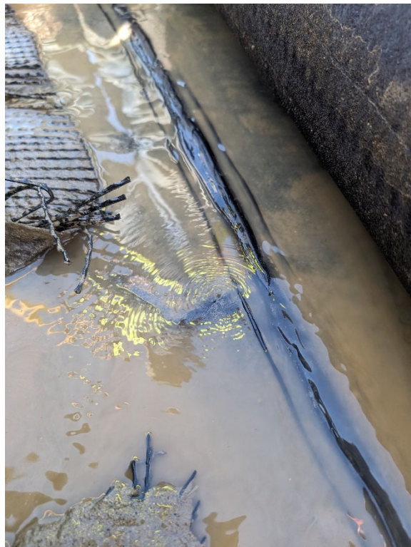
Air bubbles at the leak location
