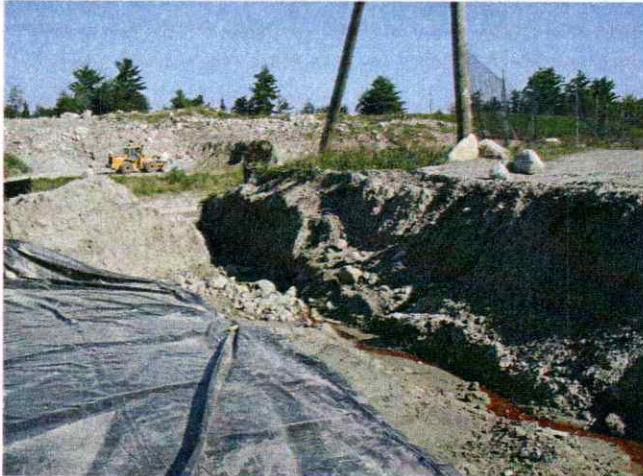
Picture 4. This picture is looking north towards MW 913M. The open trench is where the 36" culvert connecting the Stage 1 Phase 1 down chute to detention pond 3 was located.
