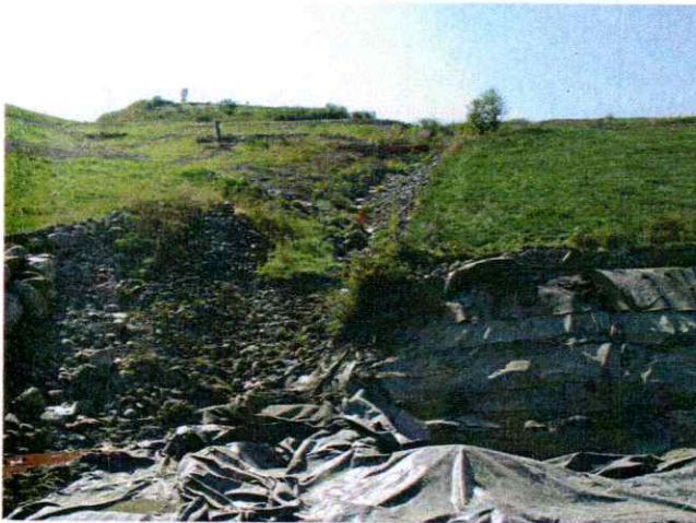
Picture 2. This picture is looking up (south) the Stage 1 Phase 1 downchute. The excavated anchor trench is to the right.
