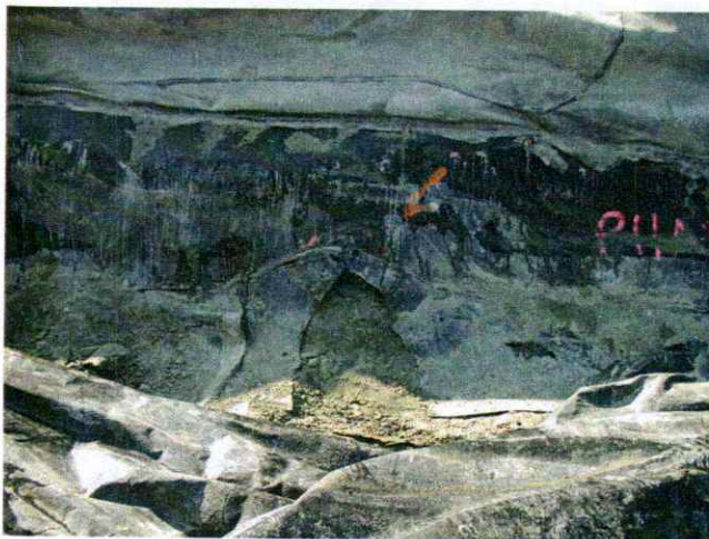
Picture 3. This picture is looking north at the Stage 1 Phase 1 anchor trench. Note arrow pointing out hole in geomembrane cap.
