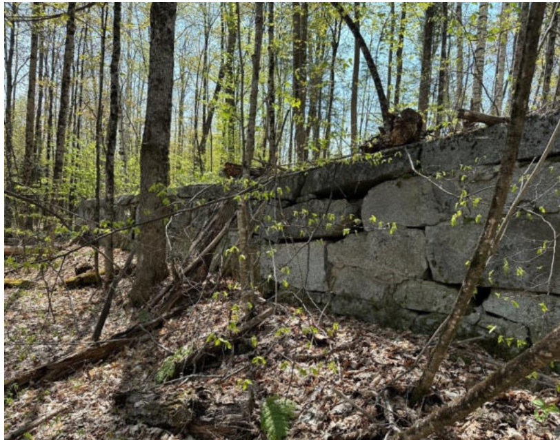
This stone foundation is in excellent condition and evidence of past dwellings. Foundations in various conditions are found throughout town. Photo taken 5-11-2023.
