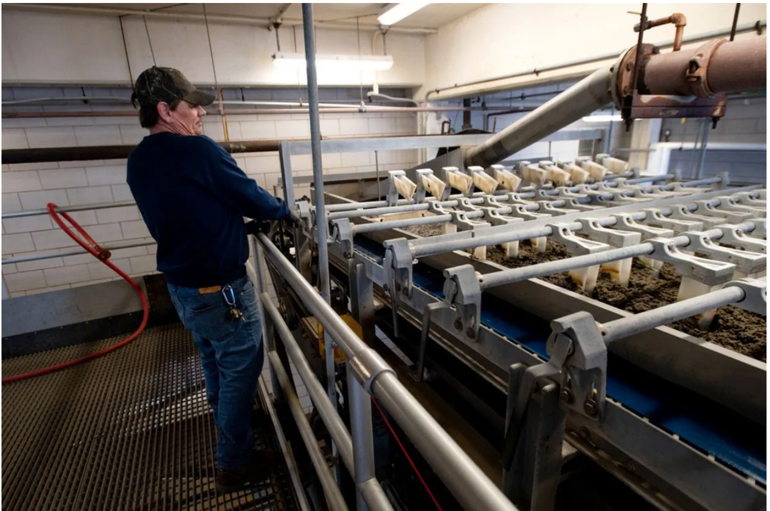
Phil Besse shakes the separators on a machine used in the dewatering process of waste at the Bangor Wastewater Treatment Plant on Main Street. Credit: Linda Coan O'Kresik / BDN
