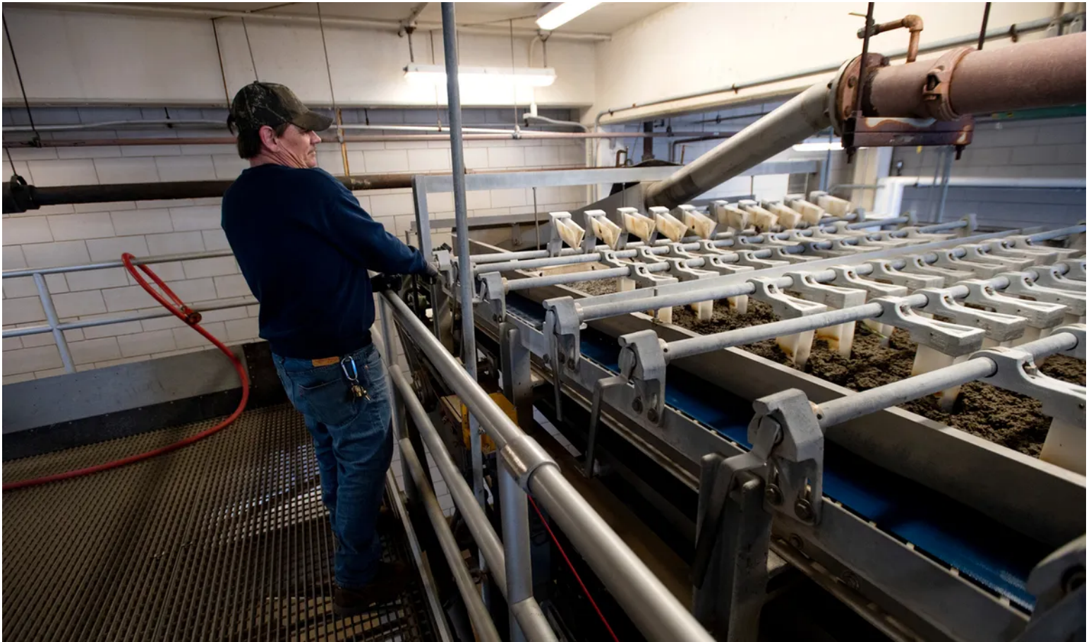
Phil Besse shakes the separators on a machine used in the dewatering process of waste at the Bangor Wastewater Treatment Plant on Main Street on March 1, 2023. Credit: Linda Coan O'Kresik / BDN
