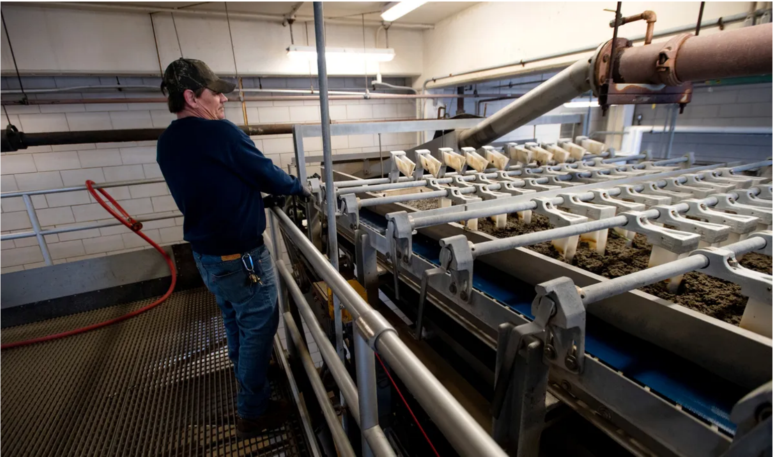
Phil Besse shakes the separators on a machine used in the dewatering process of waste at the Bangor Wastewater Treatment Plant on Main Street on March 1, 2023. Credit: Linda Coan O’Kresik / BDN
