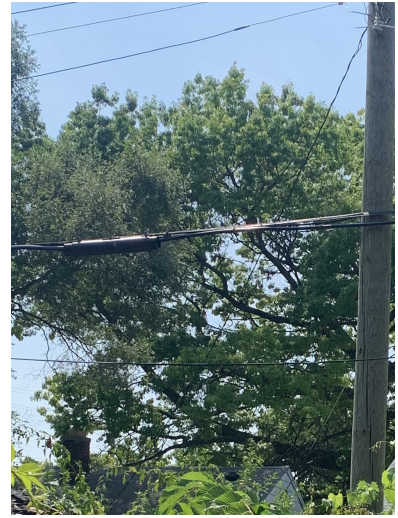
The down power line has been repaired. Fire Marshall Incident Number 21-0030820.
