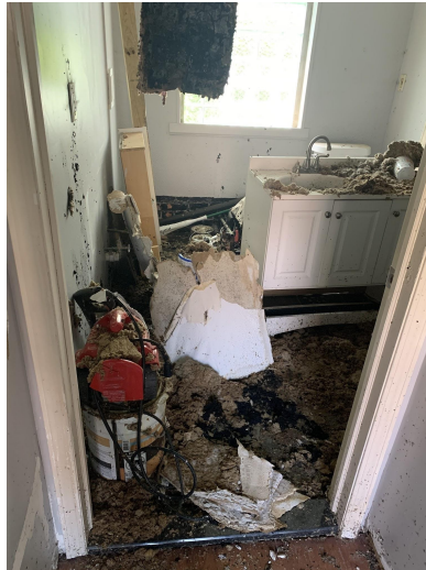
The bathroom ceiling was knocked out during the down power line.
