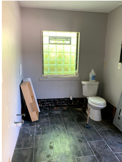
Some damage to the bathroom after the water pipes failed were unnecessary or damaged due to incomplete mitigation services. The back wall and right side were cut out during mitigation. The wall on the left was untouched.
