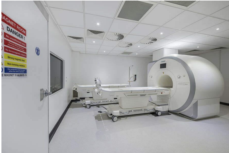
Image: MRI Scanner Room
