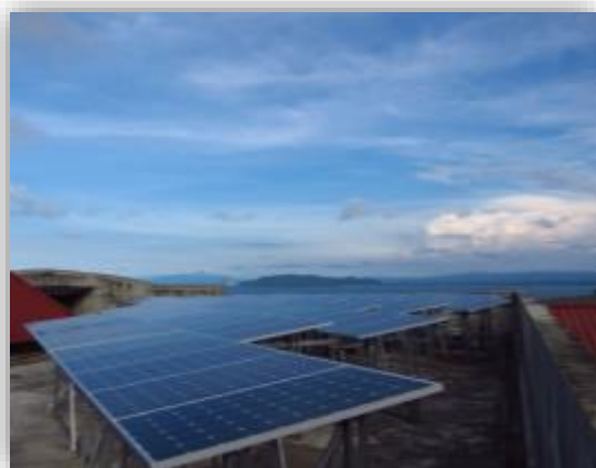
Figure 3. On-grid installation in Papua
