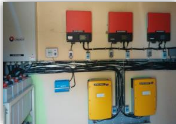
Figure 4. AC-Coupling in Loola Eco Resort
