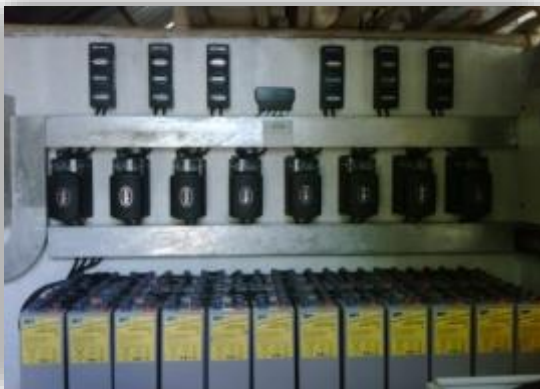
Figure 1. Off-grid installation in Nikoi Island
