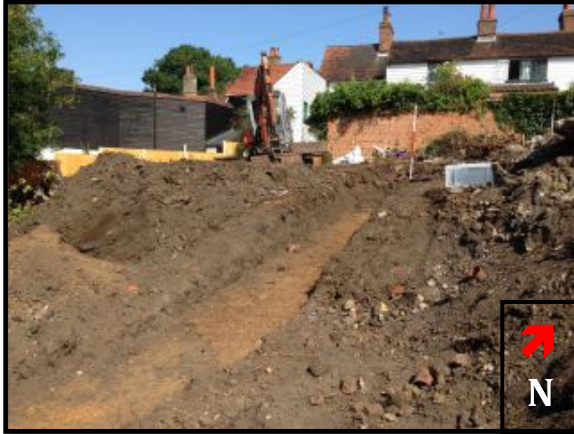
A1 - Trench 1 Direction: North - South Size: 1.2m Width x 12m Length x 0.4m - 0.7m Depth
