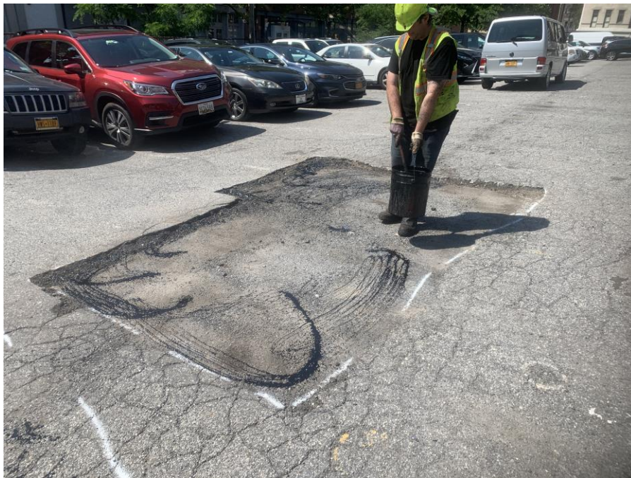
Photo 1: View of cut edges in the existing asphalt and placement of AC-5 (facing project southwest)
