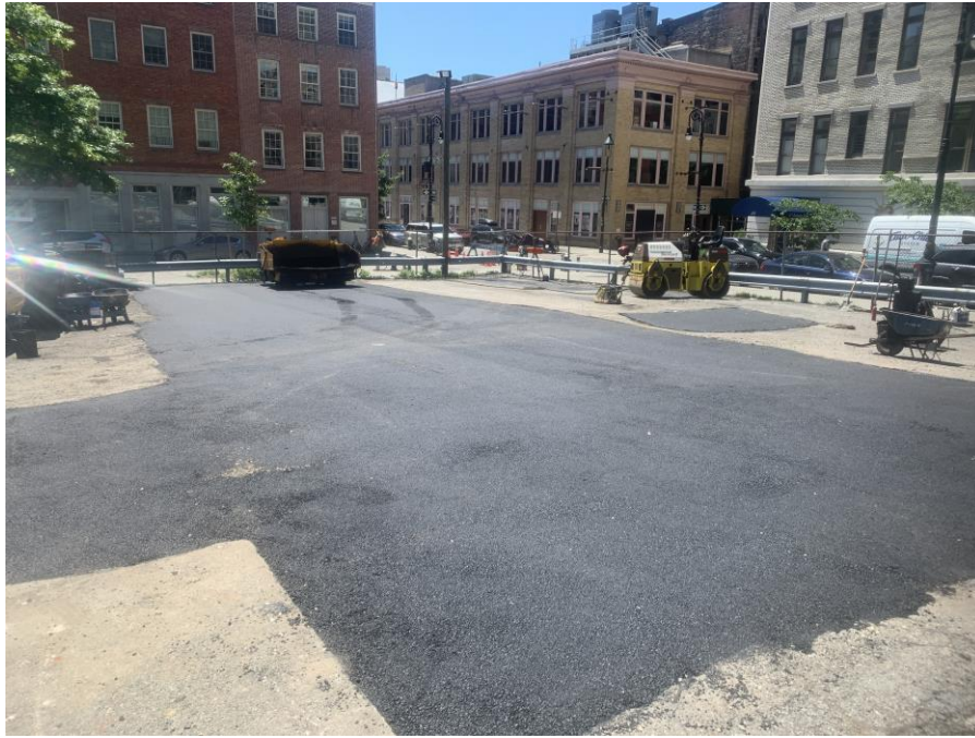
Photo 1: View of the infilled depressed areas near the corner of Water Street and Beekman Street at the end of the day (facing project southwest)
