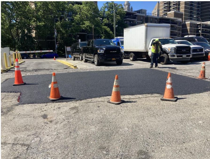
Photo 2: View of the infilled depressed areas near the site entrance at the end of the day (facing project east)
