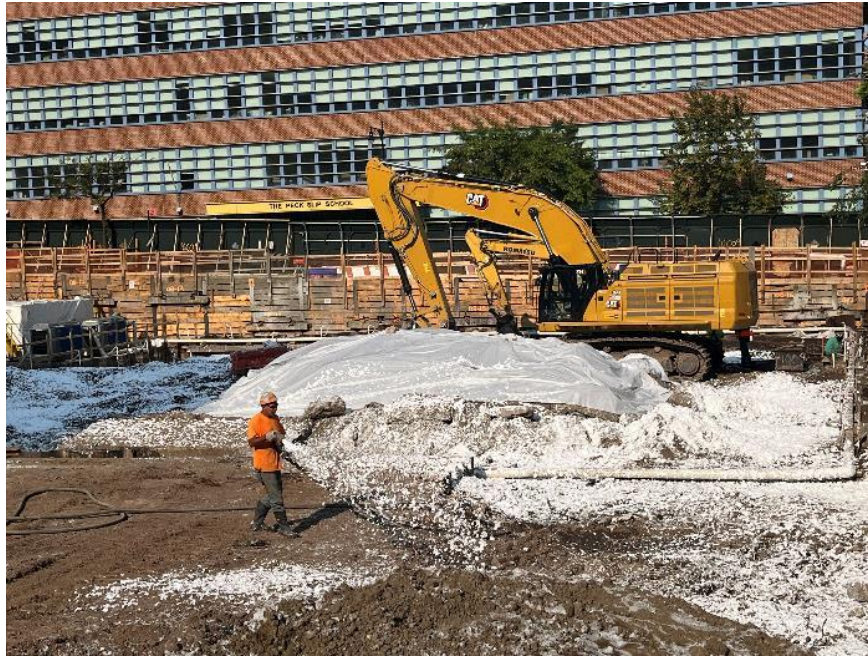
Photo 1: CCJV applying Atmos® AC-645 dust/vapor suppressing foam in the southeastern part of the site (facing east)
