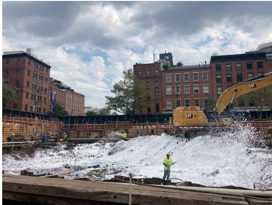
Photo 2: CCJV actively applying Atmos® AC-645 dust/vapor suppressing foam during excavation/loading in the southeastern part of the site (facing south)
