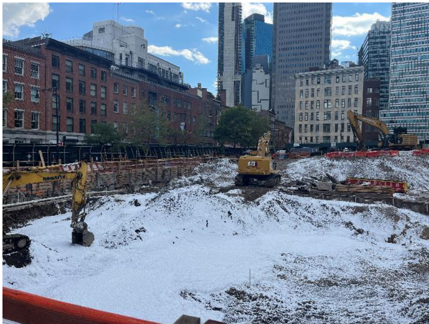
Photo 2: Atmos ® AC-645 dust/vapor suppressing foam applied to exposed soil/fill for the temporary overnight cover (facing southwest)
