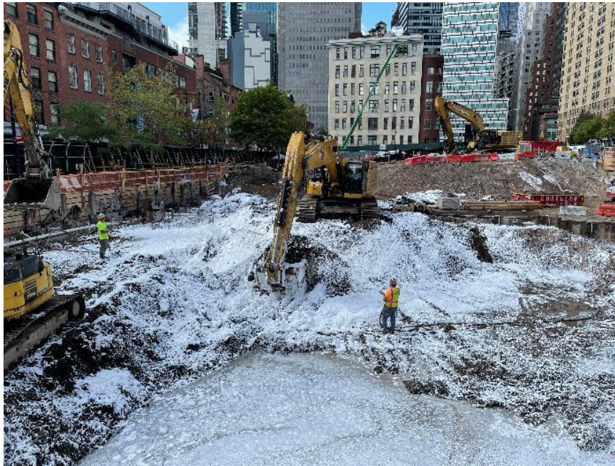
Photo 1: CCJV actively applying Atmos ® AC-645 dust/vapor suppressing foam during excavation/loading in the southeastern part of the site (facing west)
