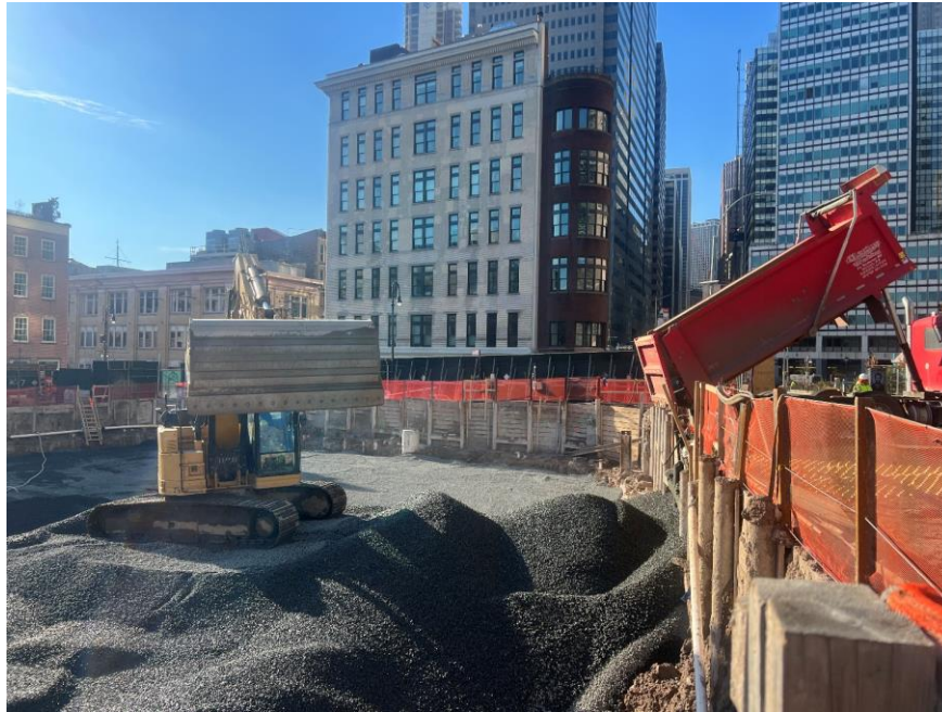
Photo 1: ECD importing 0.75-inch virgin stone for installation of a temporary site cover (facing west)
