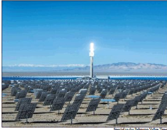
The Crescent Dunes solar plant near Tonopah.
