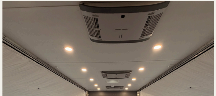
Built-In Climate Control
