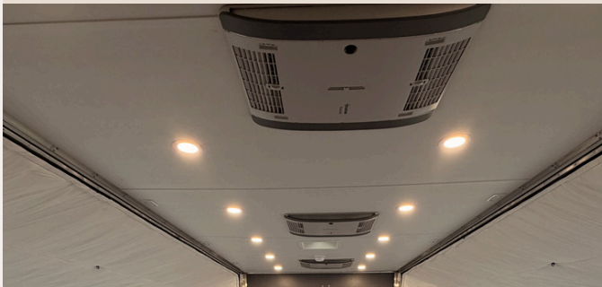
INTEGRATED HVAC, ELECTRICAL OUTLETS AND LIGHTING Three 15,000 BTU roof-mounted units.
