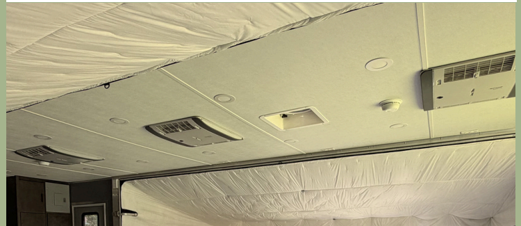
Built-In Climate Control
