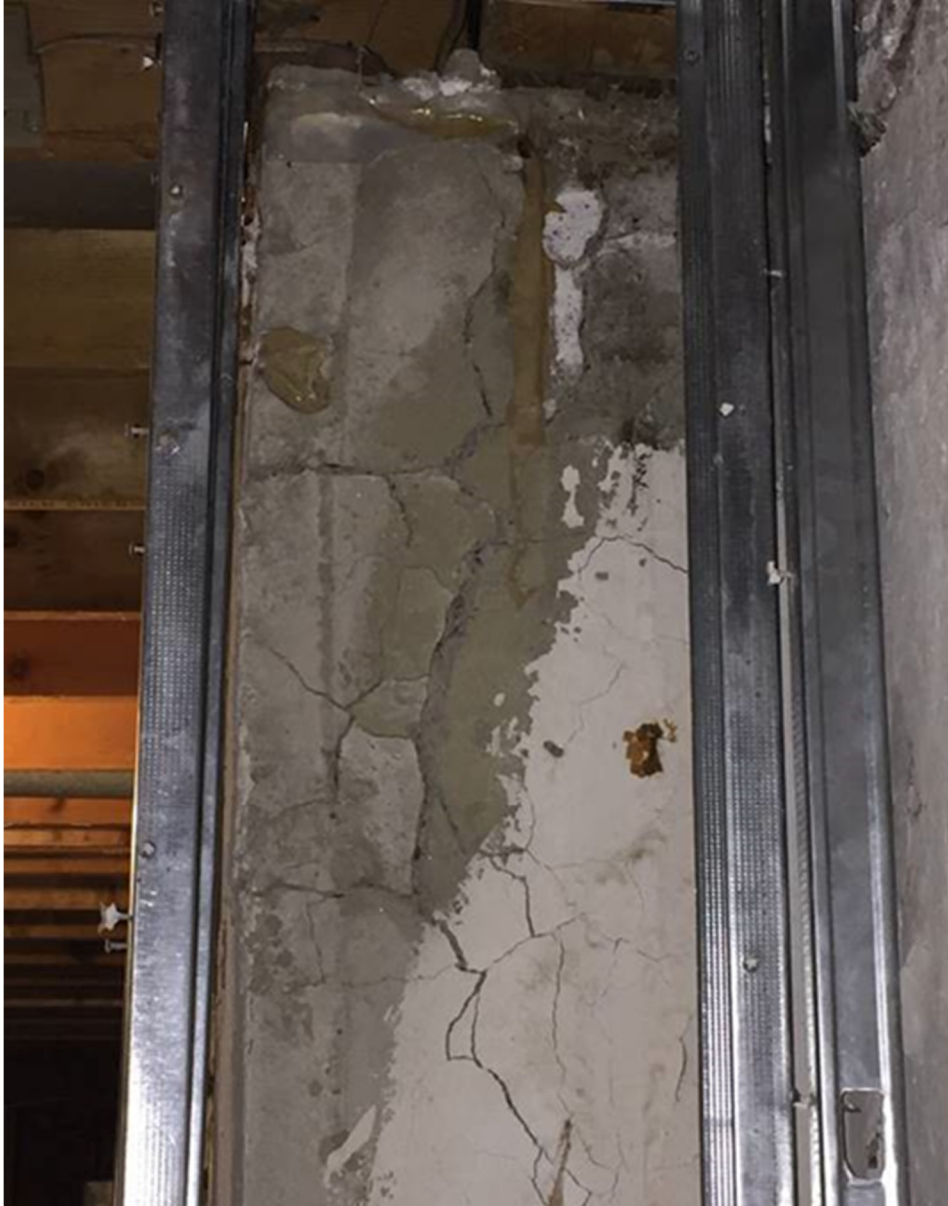
Figure 3. A crumbling foundation caused by the presence of pyrrhotite.
