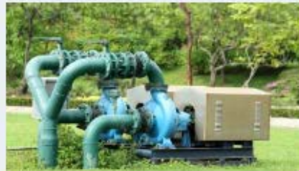
Remote Lift Station
