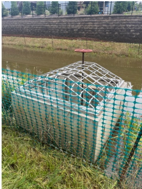
Riser of BMP2
