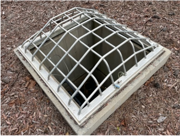
Riser of BMP3
