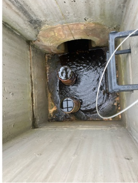
Inside riser of BMP3
