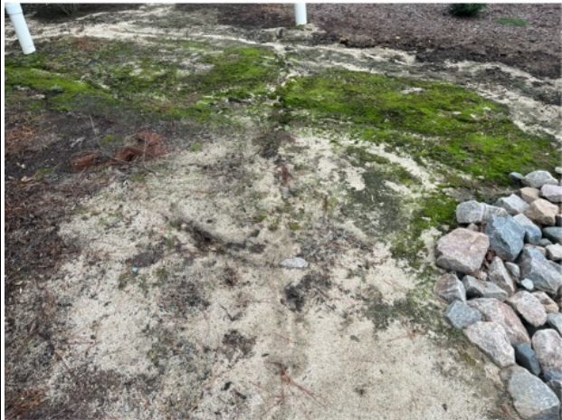
Bare areas at BMP3 basin
