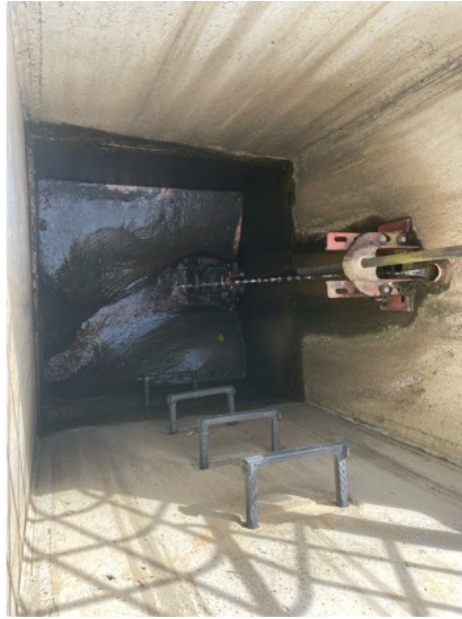
BMP2 inside riser
