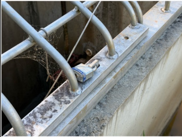
BMP 2 lock on riser
