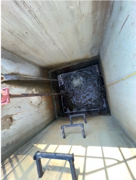
BMP1 inside riser
