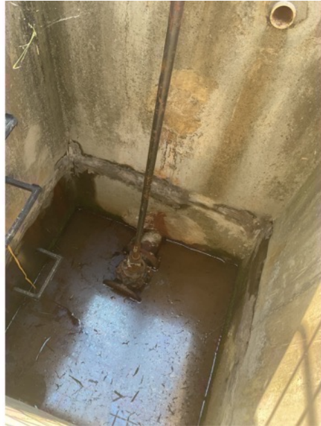
WP1 inside riser
