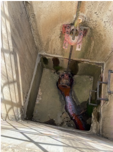
BMP2 inside riser
