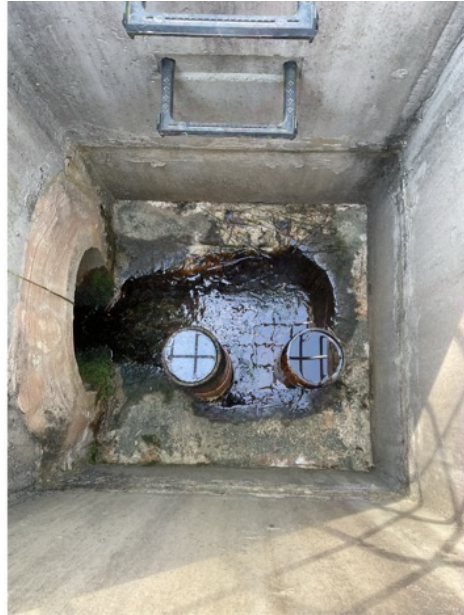
BMP3 inside riser
