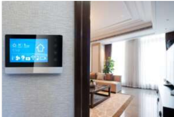
A Smart Home control panel.
