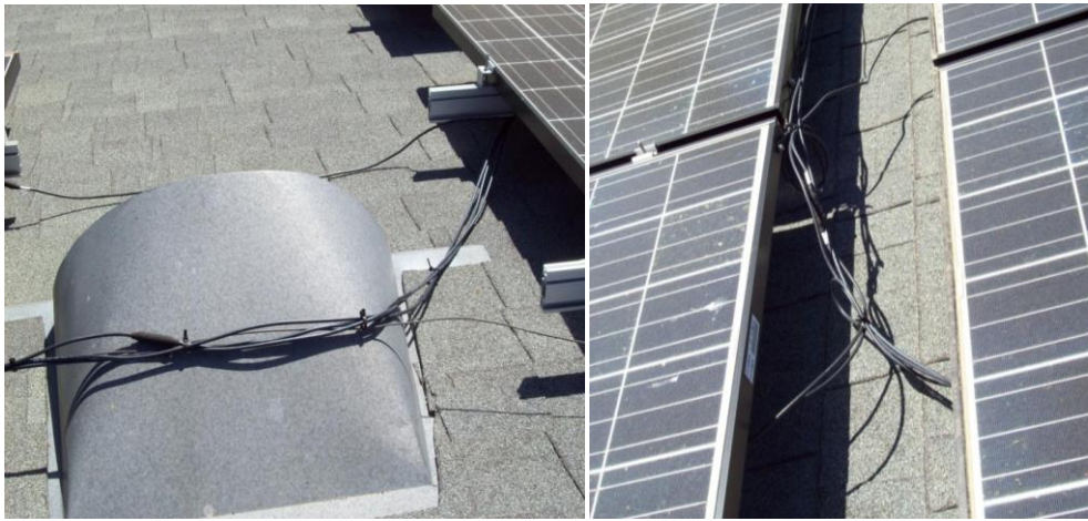
Figure 9 improper cable support with exposure to physical damage (incorrect)
