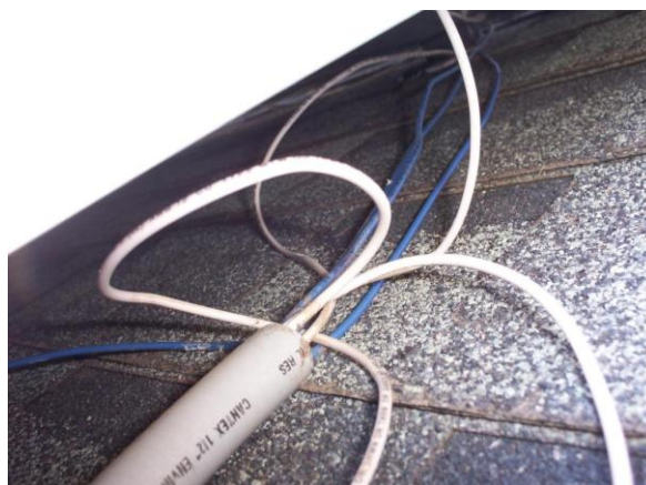
Figure 17 incorrect conductors exposed and touching roof and no strain relief (incorrect)
