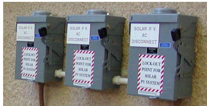
Figure 21 sign in PV ac disconnect (correct)
