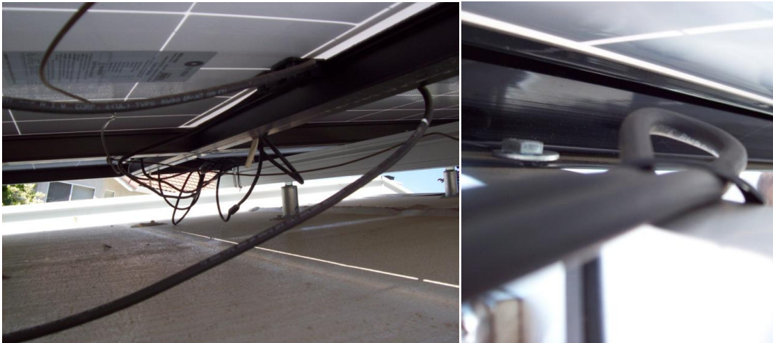
Figure 10 poor conductor handling and bending radius too tight (incorrect)
