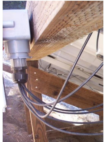
Figure 6 multiple conductors in single conductor cross-threaded cable gland (incorrect)
