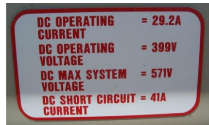
Figure 20 PV Power Source sign (correct)
