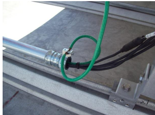
Figure 4 conductors properly protected by raceway with grounding bushing (correct)-should be secured within 12 inches of fitting (not shown)
