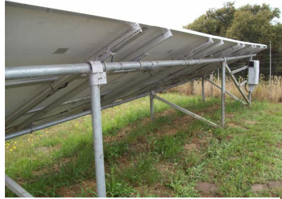
Figure 18 typical ground mount system with readily accessible wiring (incorrect)
