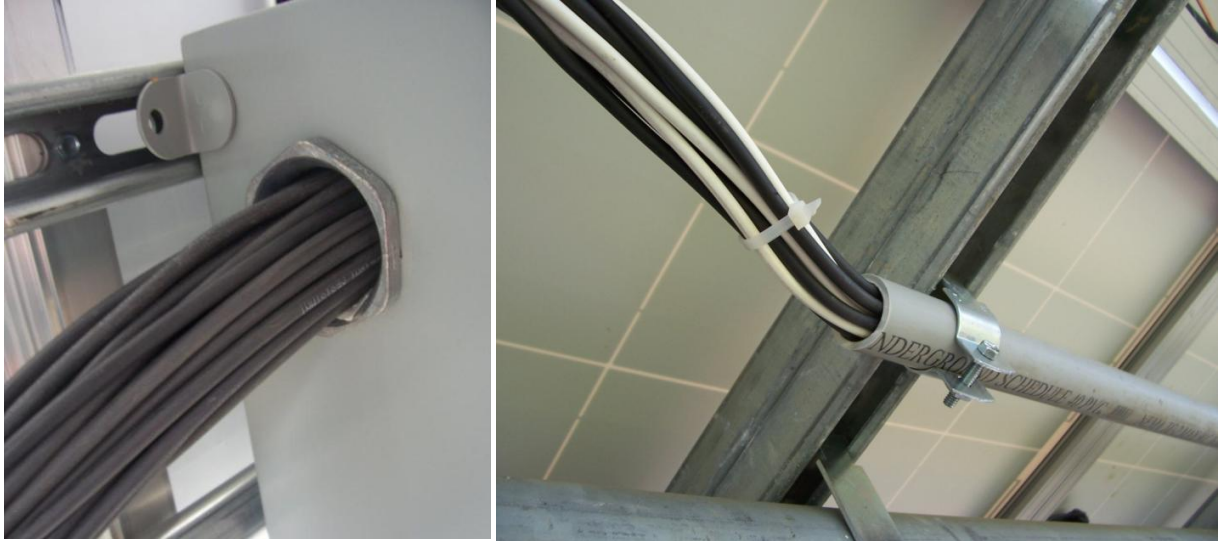
Figure 11 improper use of chase nipple and exceeding conduit fill with no end fitting (incorrect)
