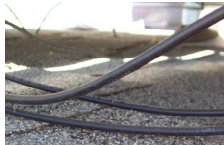
Figure 3 USE-2 conductors touching roof surface
