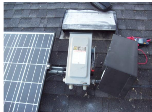
Figure 13 incorrect NEMA 3R disconnect on sloped roof designed for vertical mounting only
