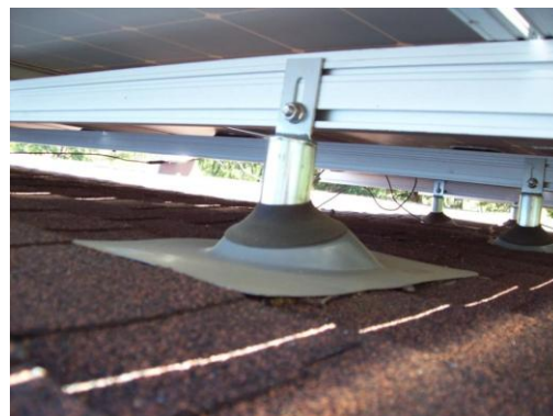
Figure 16 uninstalled flashing (incorrect)
