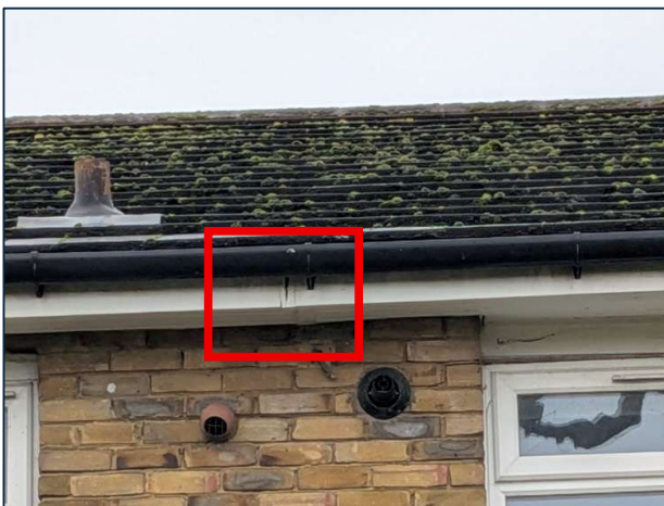
Photo 9: Split visible on join between fascia boards.
