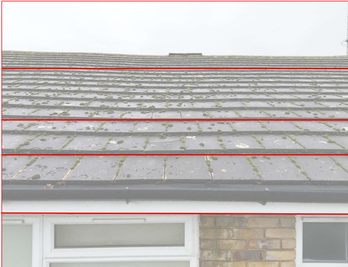
Photo 10: Straight lines drawn to demonstrate the deflection of the roof tiles.
