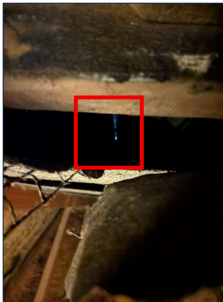
Photo 15: Example of light shining through tile joint
