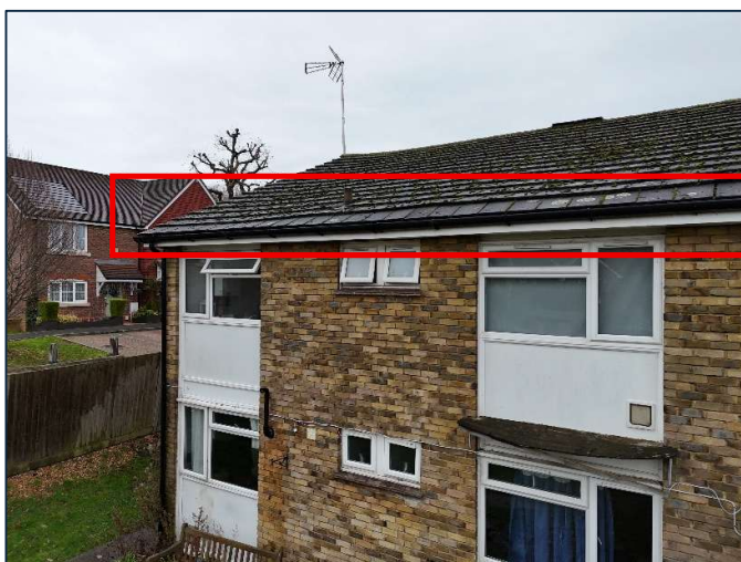
Photo 11: Bottom course of tiles with inconsistent alignment.
