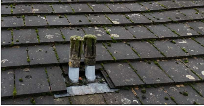
Photo 7. Example of inadequate lead detailing around (asbestos containing) cowls
