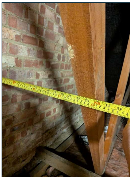
Photo 13: Distance between masonry wall and rafter
