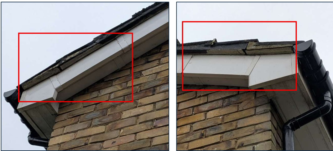
Photo 8: Deficient under cloaking and deteriorated mortar joints.
