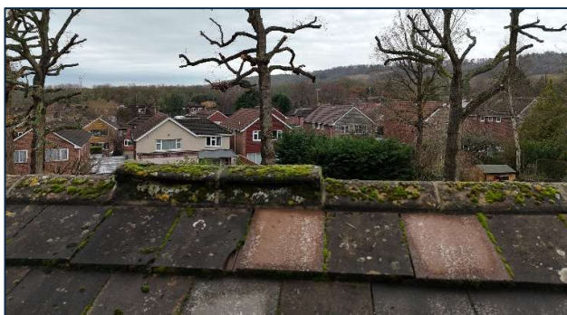
Photo 5. Defective Ridge Vent
