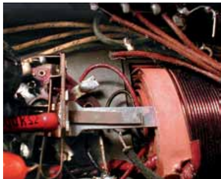
Fig.39. Removable & repairable spring loaded mains switch held closed by low temperature solder. Fits in pocket between transformer windings.
