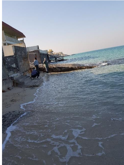
Fig. 2. Beach houses near shore line in Bnaider, Kuwait at Latitude 28° 45' 14.36" and Longitude 48° 19' 54.73" captured on 5 Dec 2017.
