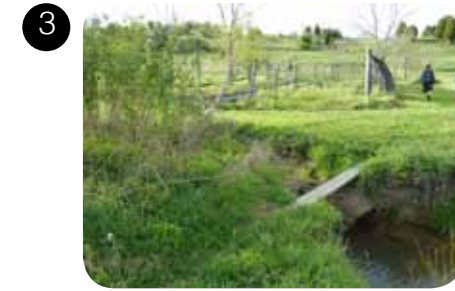
Main Hollow Creek divides the property. Crossings connect the two sides over this deeply incised stream bed, which floods several times a year.
