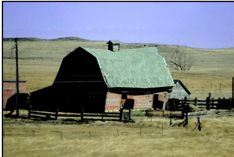
Lots of leaners in this State. Leaning barns, towers, houses, outbuildings. Guessing that comes with the windy, snowy territory.
